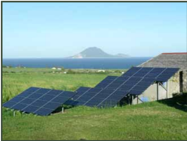
Island Energy System on St. Kitts, West Indies
