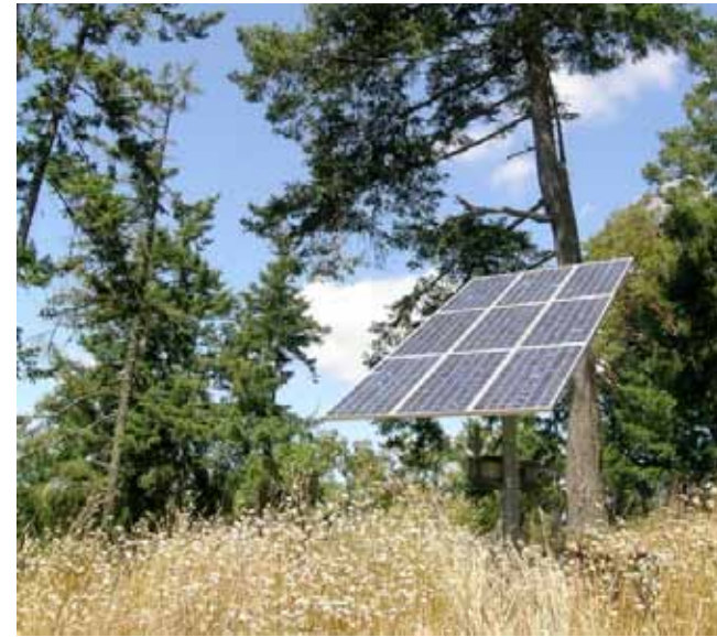
Grid-tied PV system on Orcas Island, WA
